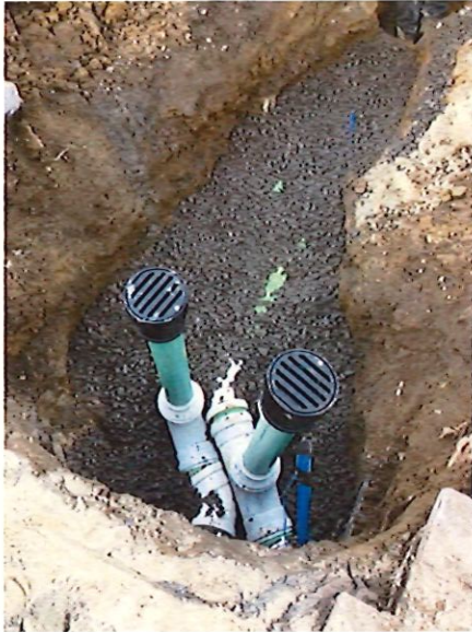
Figure 2: View of cleanouts
