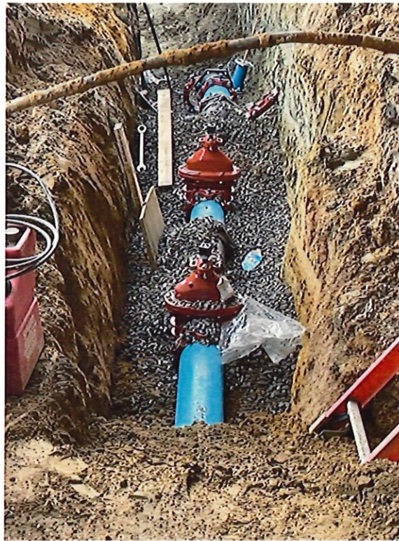
Figure 1: View of 8" gate valve, 8' to 12" Tee, and 8" gate valve for zone isolation
