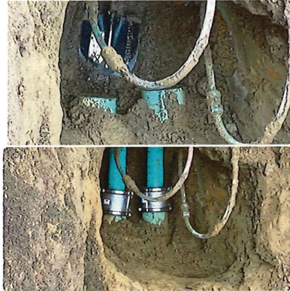
Figure 3: View of two 4" laterals at tie in point at the sewer main
