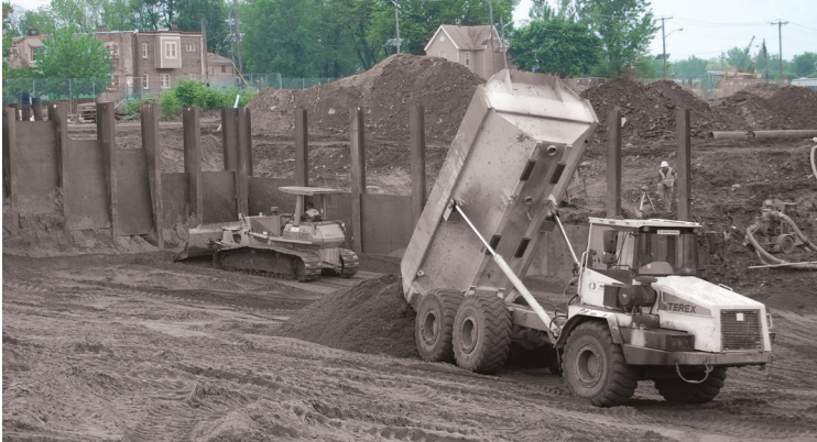
A construction crew levels the ground for the foundation of the Kroc Center.
